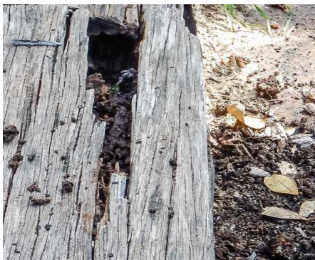
Older timber from LHI showing termite damage
