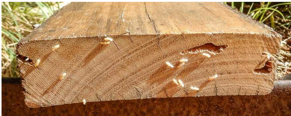
Decking from LHI showing termites and 'galleries' (damage on end of timber)
