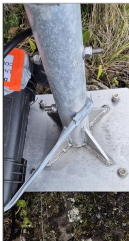
Figure 3. Image of repeater base plate and mount system.
