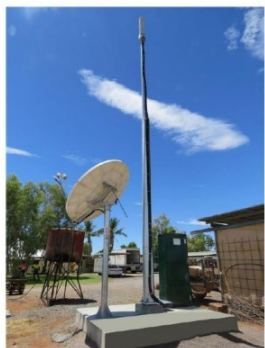
Example of a Satellite Small Cell mounted on the skid with a 9m structure
