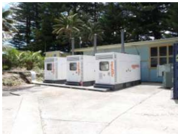
Figure 160 Three portable generators installed on a site at rear of Powerhouse following the fire in that building in November 2009. (Photo: Chris Betteridge, 2 December 2009)
