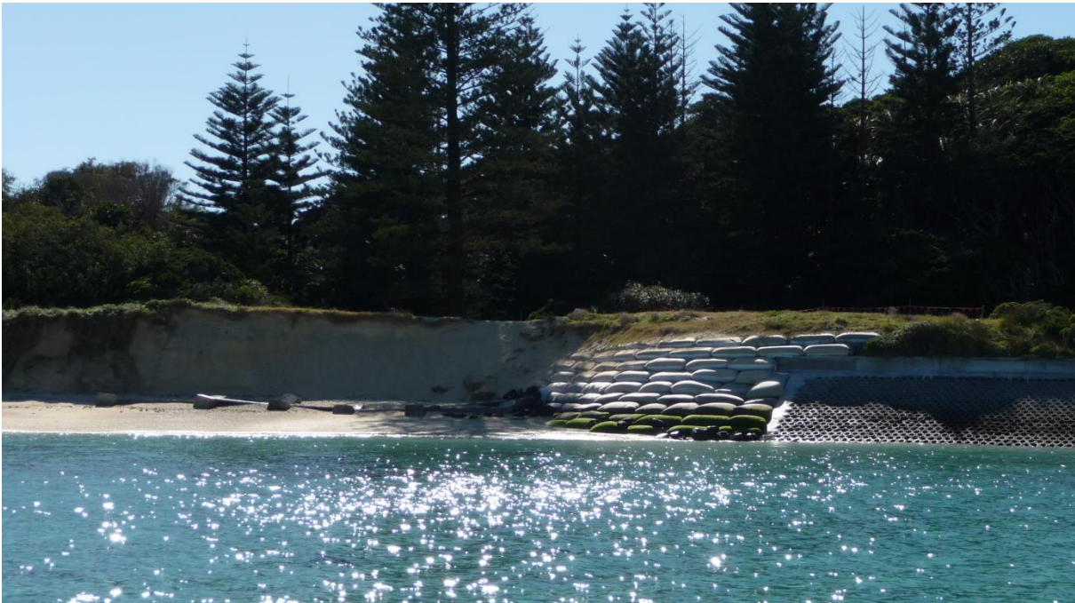
Figure 7: View (left to right) of eroding dune with concrete and rock on beach, sand-filled geotextile container wall and Seabee revetment (29 August 2012)
