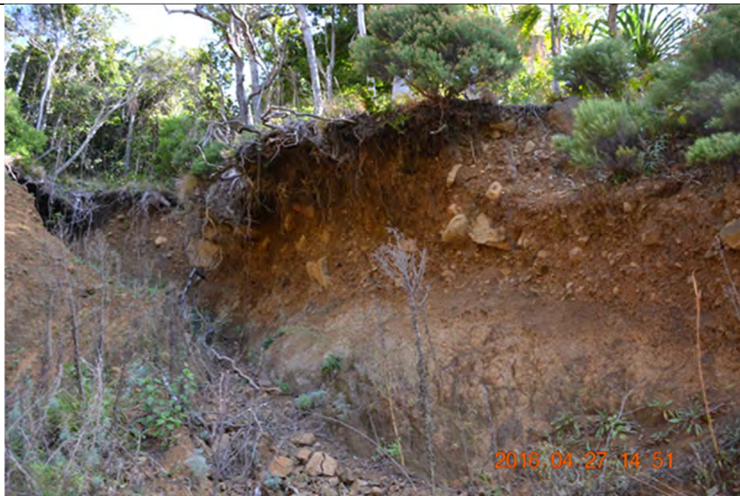
Site 9 View from backscarp area of southe western batters from top of bank
