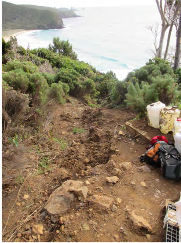
Photo 7 – Erosion channel formed in the vicinity of the walking track showing dislodged construction materials.
