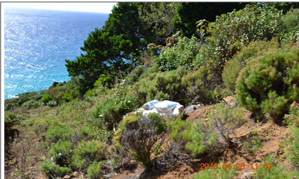
Site 5 Lower mid slope area of slide looking upslope to the north east towards toe with building materials from previous proposed works in foreground
