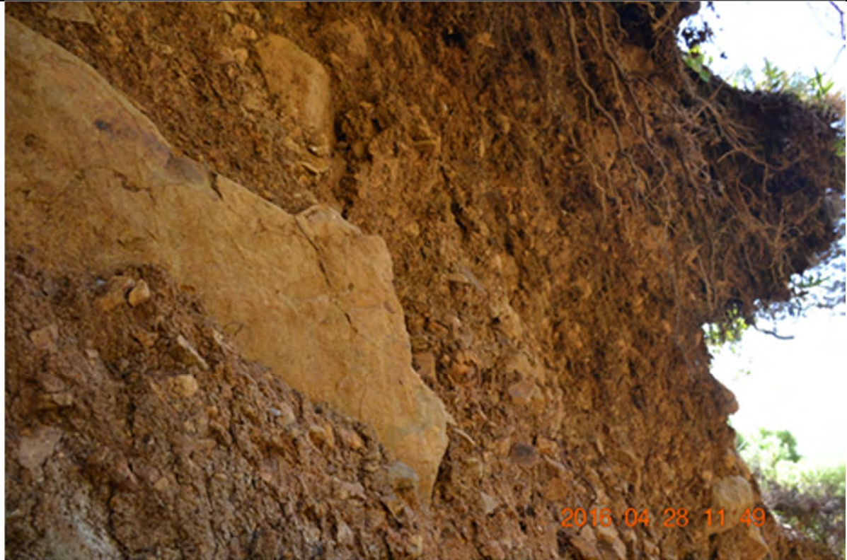
Site 8 Close up of clolluvial batters with large floaters that could detach downslope towards track.
