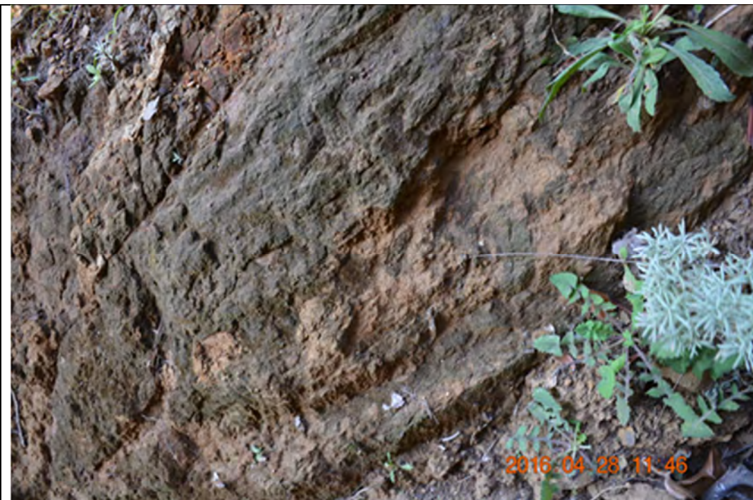
Site 8 Exposed floor of Upper slope section of slide showing extremely weathered outcrop of very weak basaltic dyke with soil like fabric and strength
