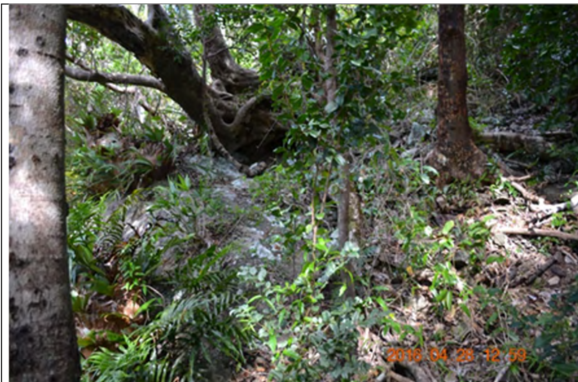
Site 10/ 11/12 Typical View of hard basalt rock outcrop about 20m upslope of slide
