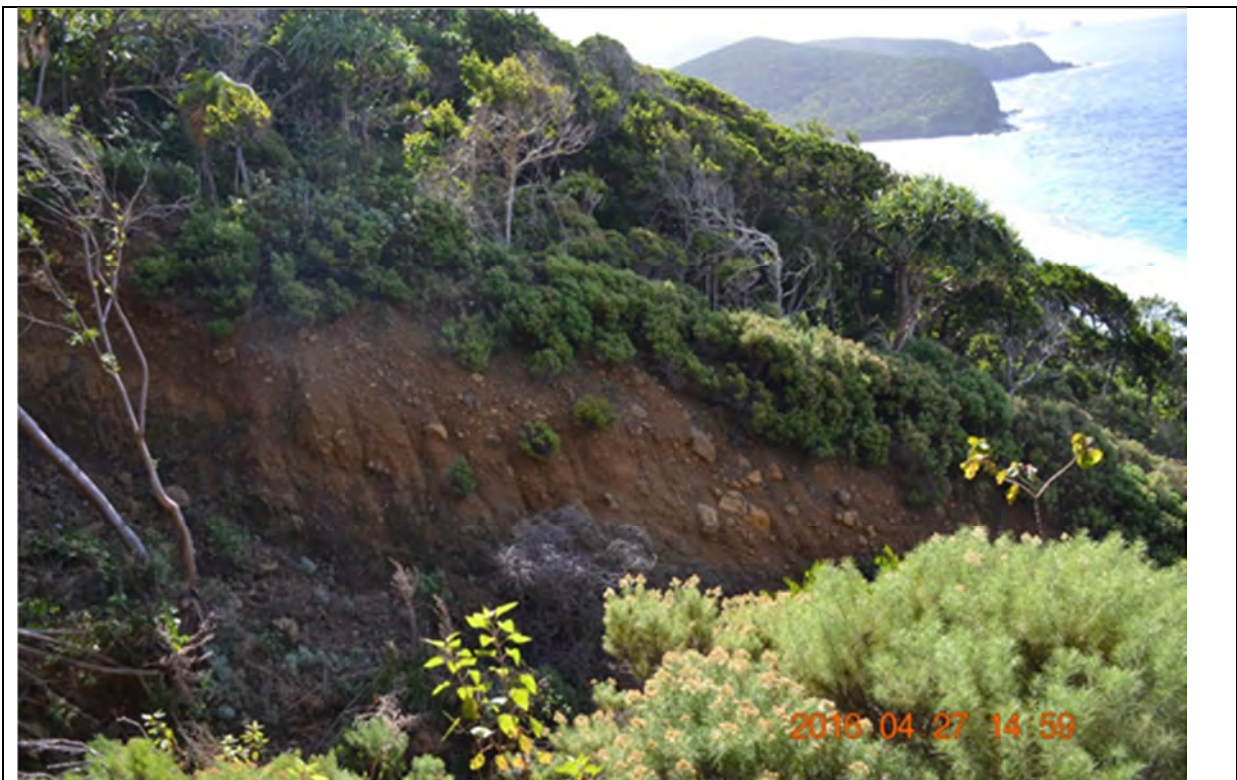
Site 9 View from backscarp area of western batters from top of bank further downslope
