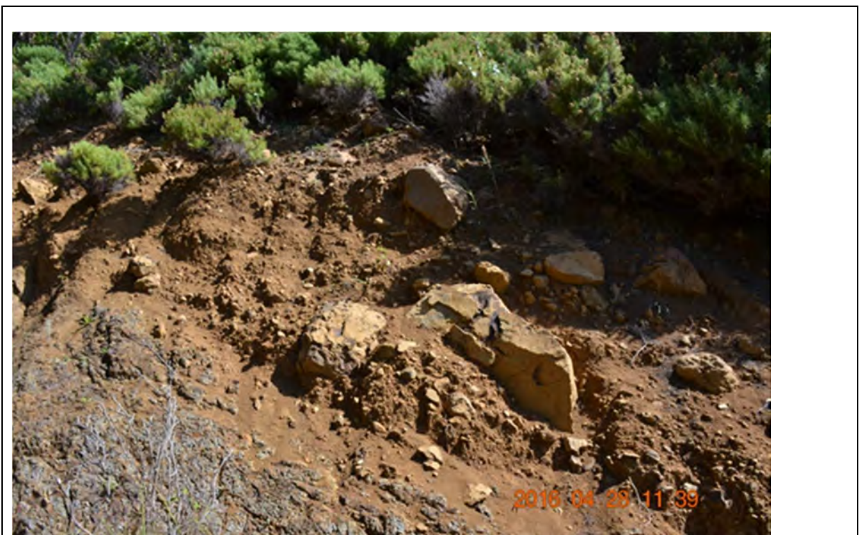
Site 7- Mid to upper slope area looking north west to exposed colluvial batters with large rock "floaters" that could detach down slope towards the track
