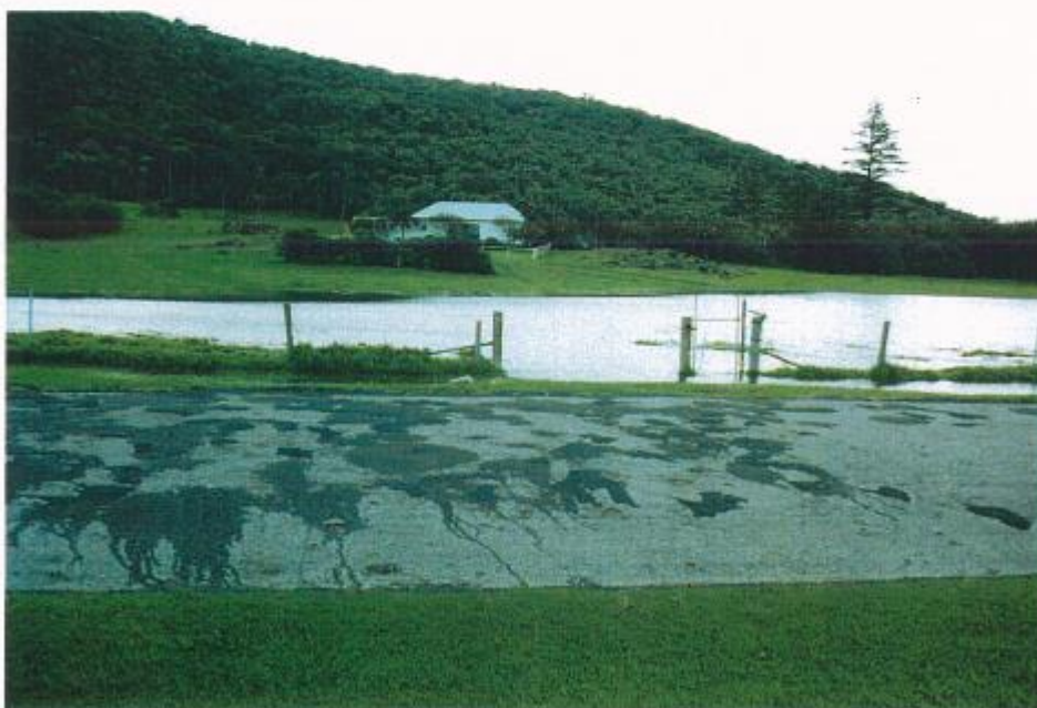
Photograph 10: Ponded area in front of Mr S Fenton June 1996
