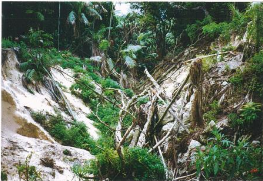
Photograph 20 : Typical land slip initiation near Clear Place
