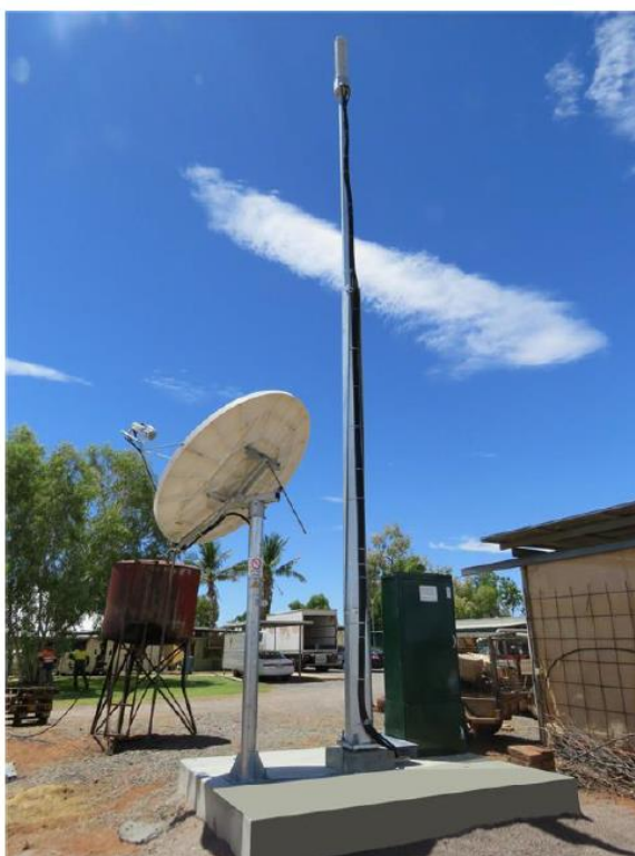
Example of a Satellite Small Cell mounted on the skid with a 9m structure
