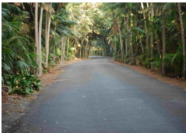
Lagoon Road. Note absence of side drains.
