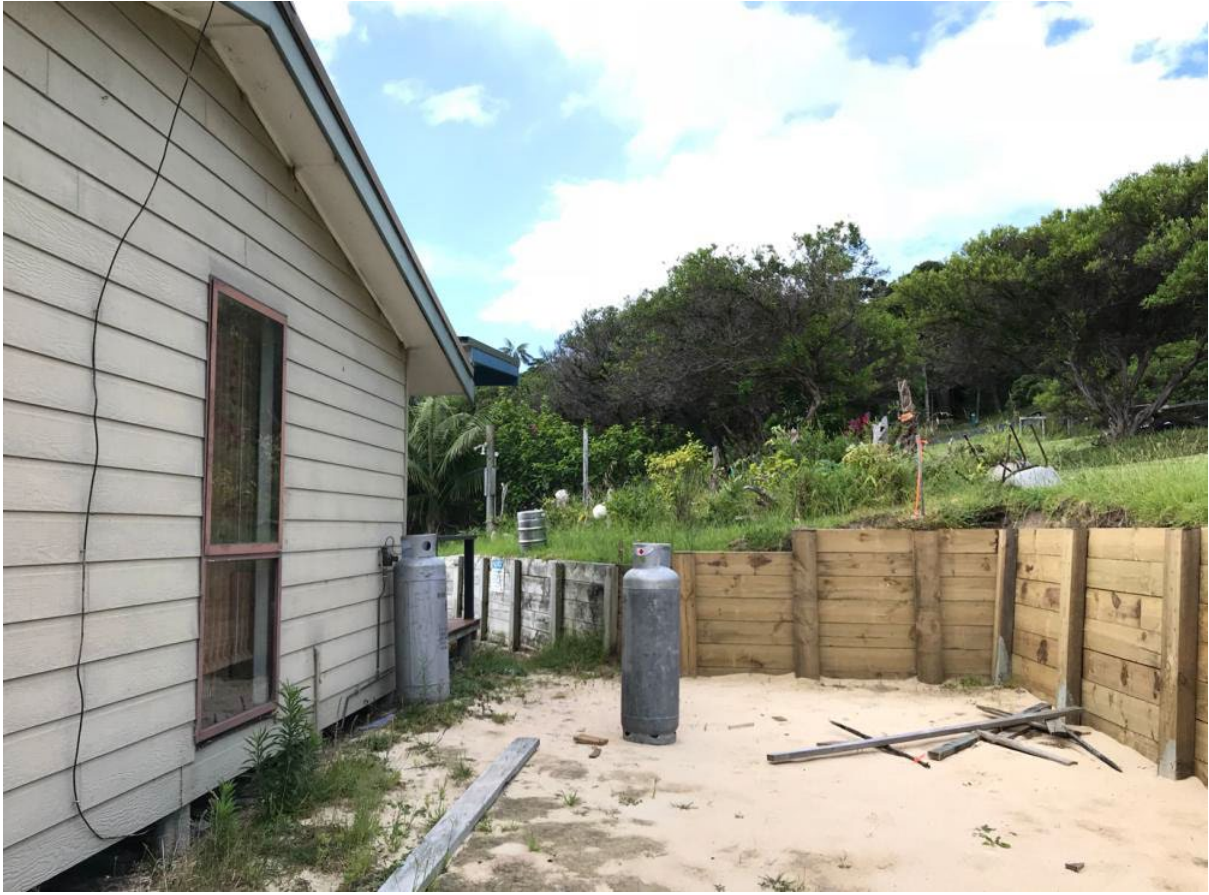
Above and below: Proposed area for ground and first floor additions, showing constructed retaining walls
