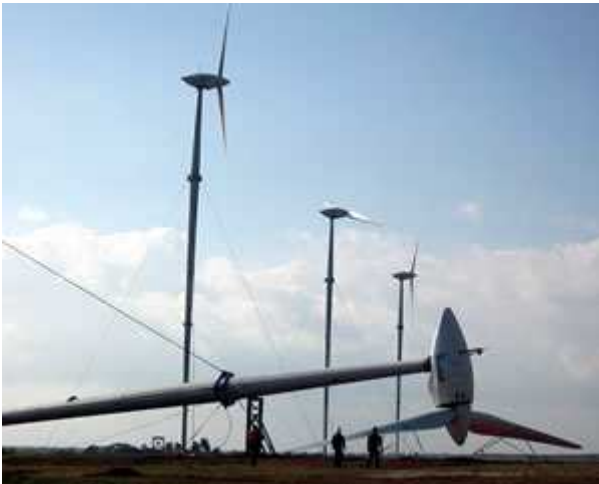
Figure 7: Vergnet MP 275kW wind turbines 10
