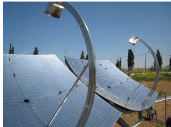
Figure 5: Concentrating PV Array– Dish
