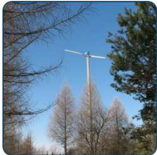
Figure 8 - WES18 (Lagerwey 18/80) Wind turbine
