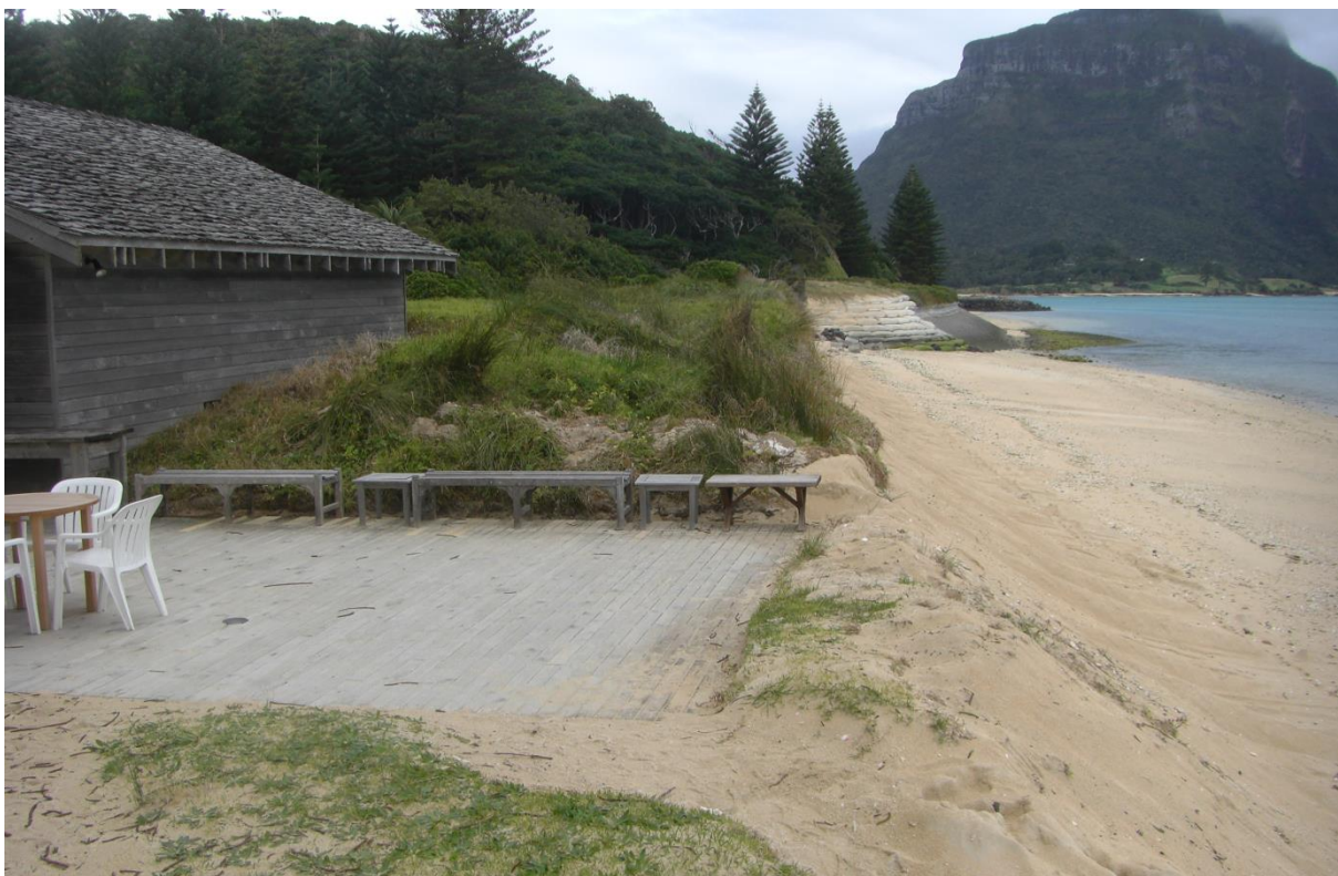
Figure 38: Erosion escarpment adjacent to deck at Pinetrees boatshed in August 2012
